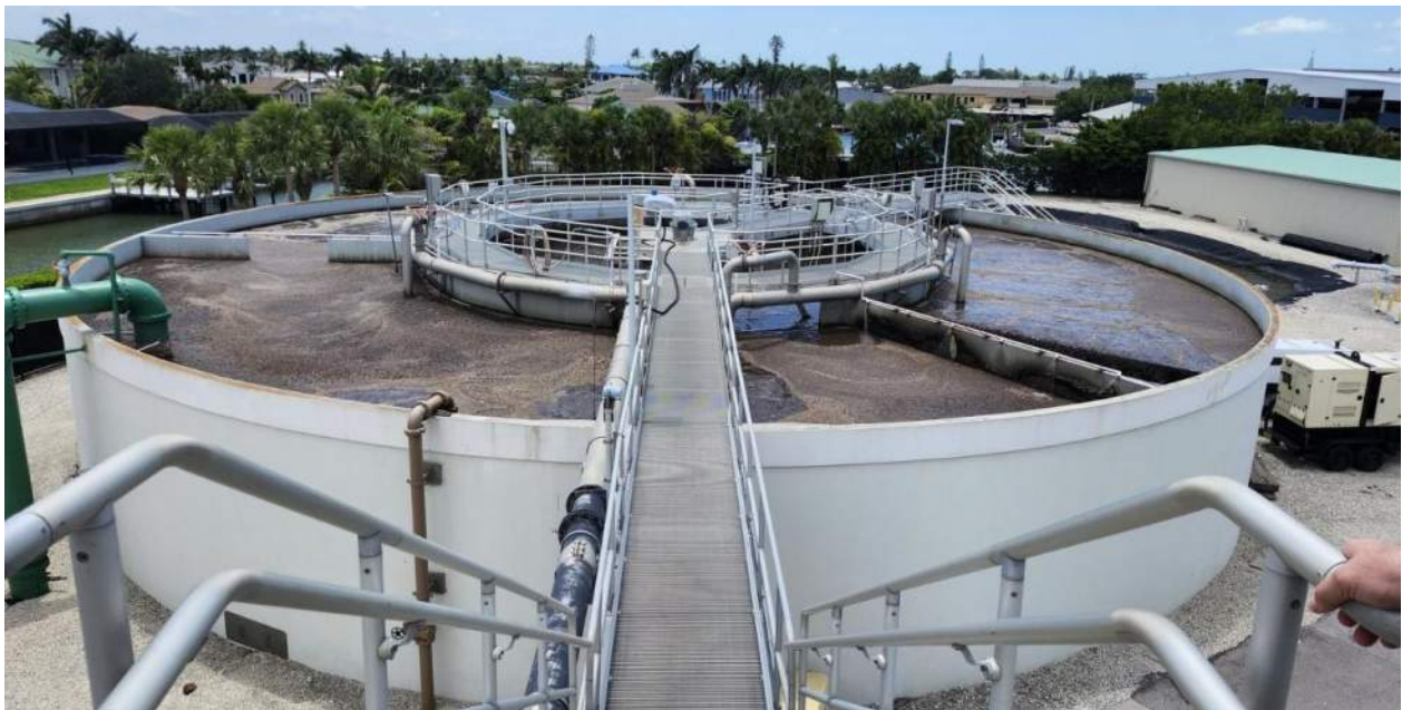
Figure 3-1 Existing MLE Tanks
