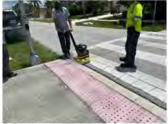
Whiteheart Ave. Trip Hazzard Removal.
